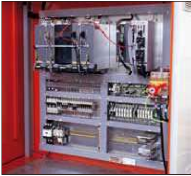
High-tech electrical cabinet meets the latest CE regulation.
